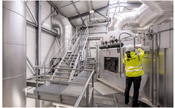
Exemplary boiler house of a GETEC biomass plant.
